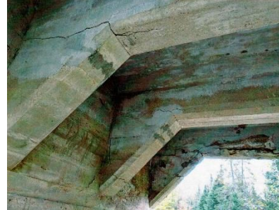
South Span Connection - cracks
