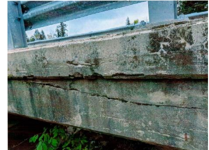
West Fascia South End Cracks
