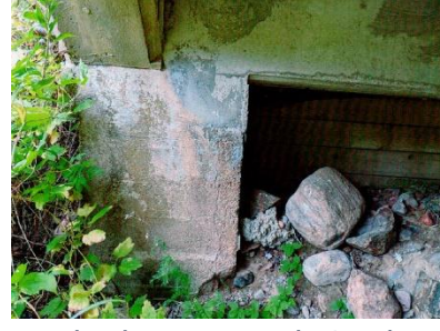
North Abutment with Crack
