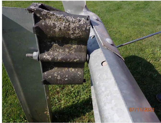
Photograph No. 4: 0020: Detached post at southeast corner.
