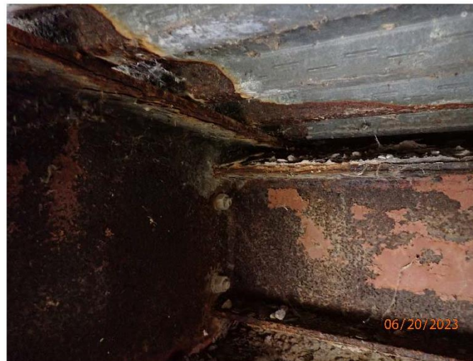
Photograph No. 4: 0778: Area of severe corrosion on west exterior girder.
