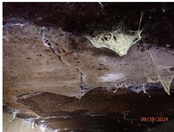
Photograph No. 4: 0449: Area of failure in concrete arch at west end of structure.
