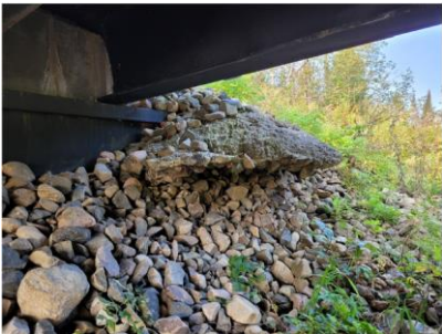
Undermining at Southwest Corner
