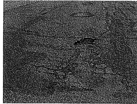
Photo 67 - Asphalt failure on Leeville Drive
