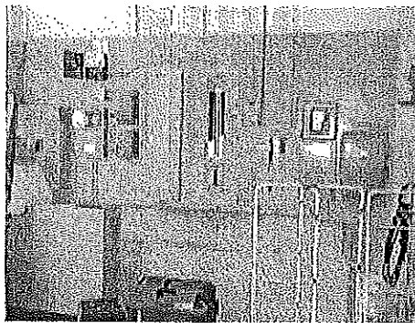
Photo 58: Pool Bldg. – Electrical Panels
