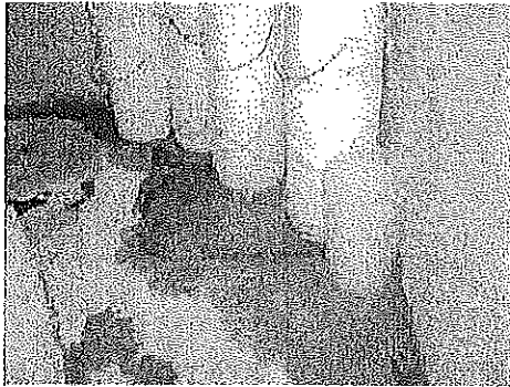
Photo 42: WTP – Basement Alum Tank
