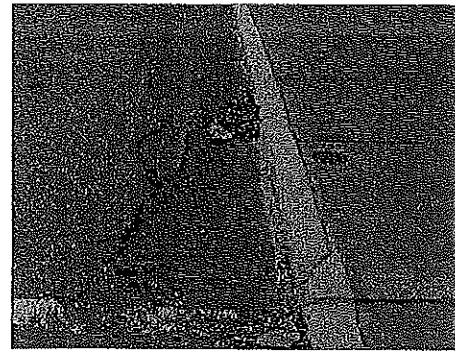
Photo 71 - Curb height diminished on 3 rd Avenue E
