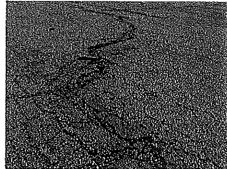
Photo 79 - Deep asphalt cracking
