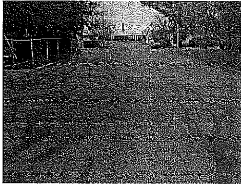
Photo 66 - Severe alligator cracking on 2 nd Street E
