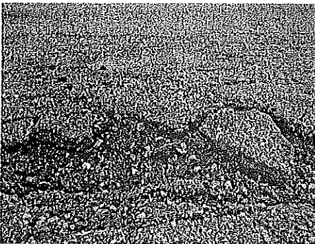
Photo 80 - Severe asphalt failure
