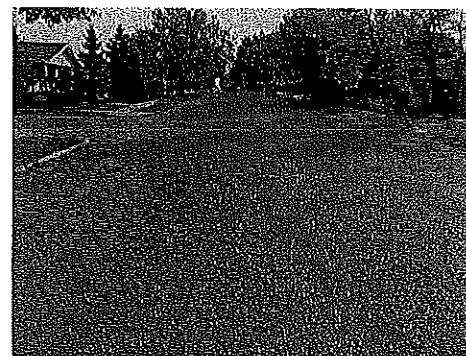
Photo 73 - Surface spalling occurring along watermain on 6 th Avenue E
