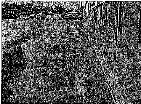
Photo 68 - Asphalt built up causing water to pool in roadway On Centre Street
